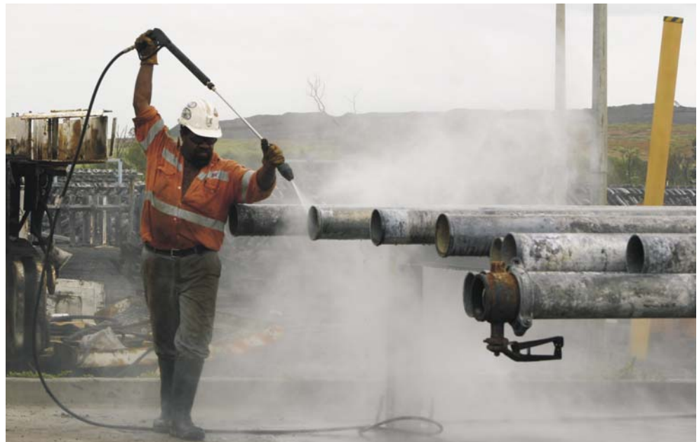
George Tonga, an employee with G & S Engineering, refurbishing water pipes at Moranbah North. This work is carried out on a purpose-built facility which allows the task to be performed safely and the waste material to be contained.
